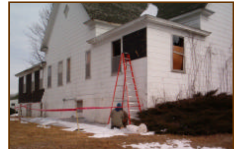
This recent AHEAD, Inc. demolition managed by Area 15 RPC requires asbestos abatement. Here the workers are carefully removing slate siding containing asbestos and bagging each piece as they proceed. Workers are equipped with respirators.
