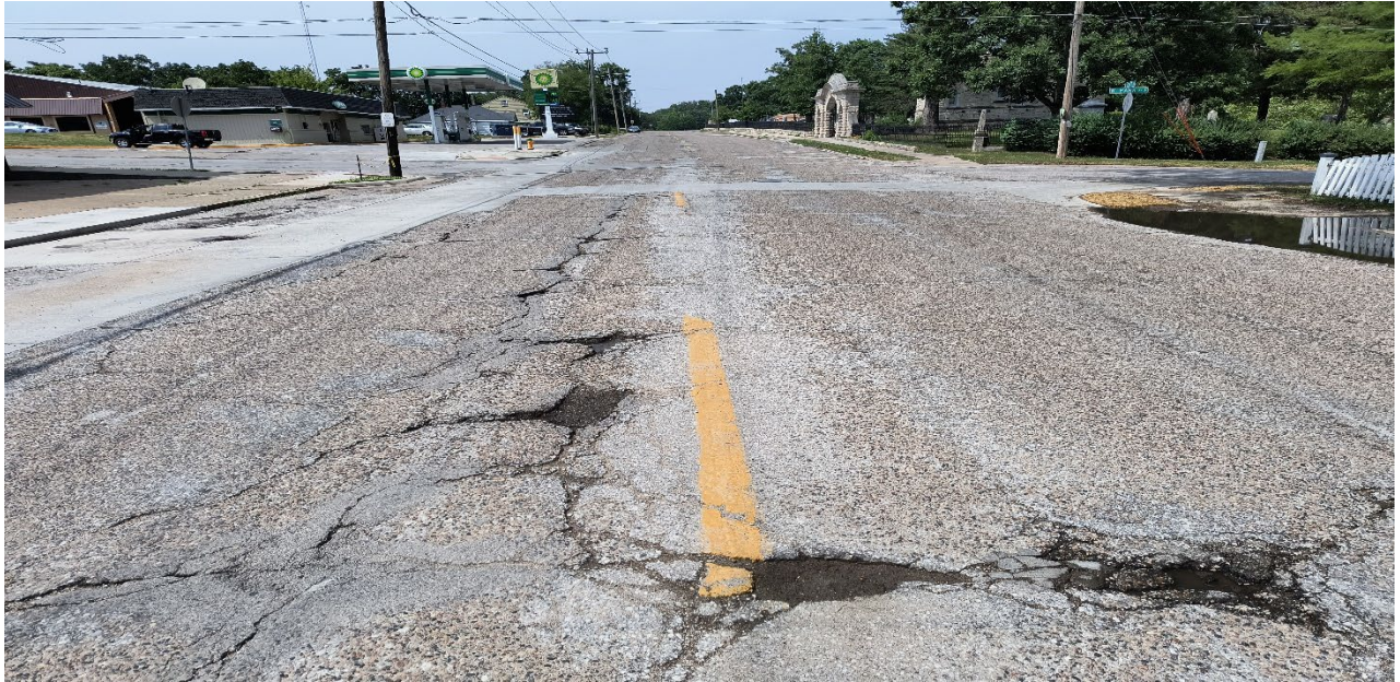
North Court: This form of deterioration can be found throughout the project.
