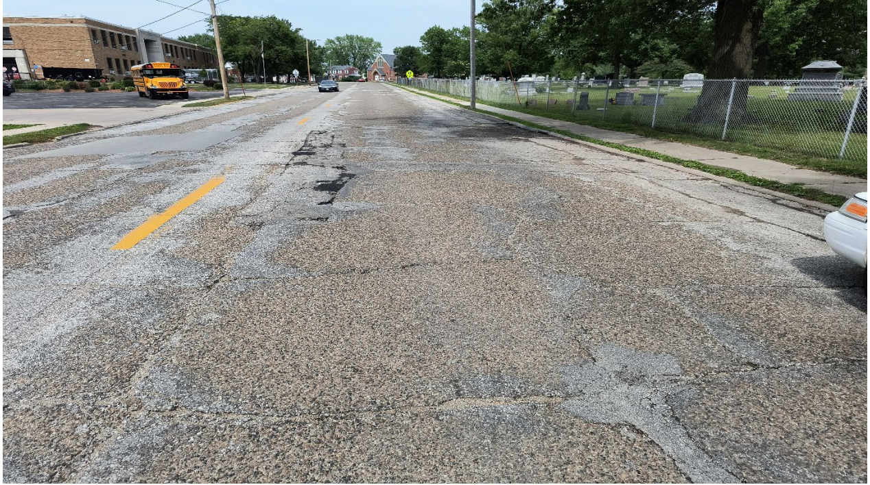
Existing Street Condition:
