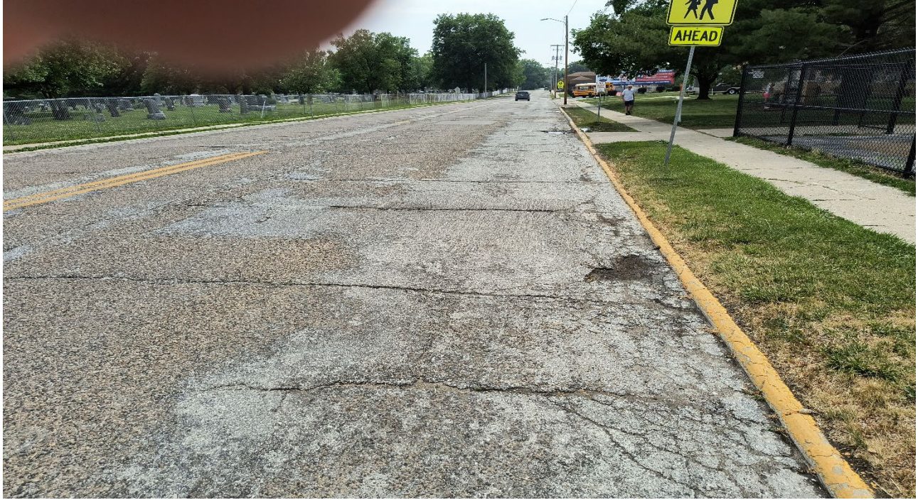
Gutterline failure, existing pavement condition.
