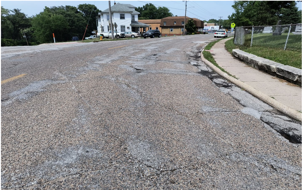
Failing gutterline. Pavement deterioration.
