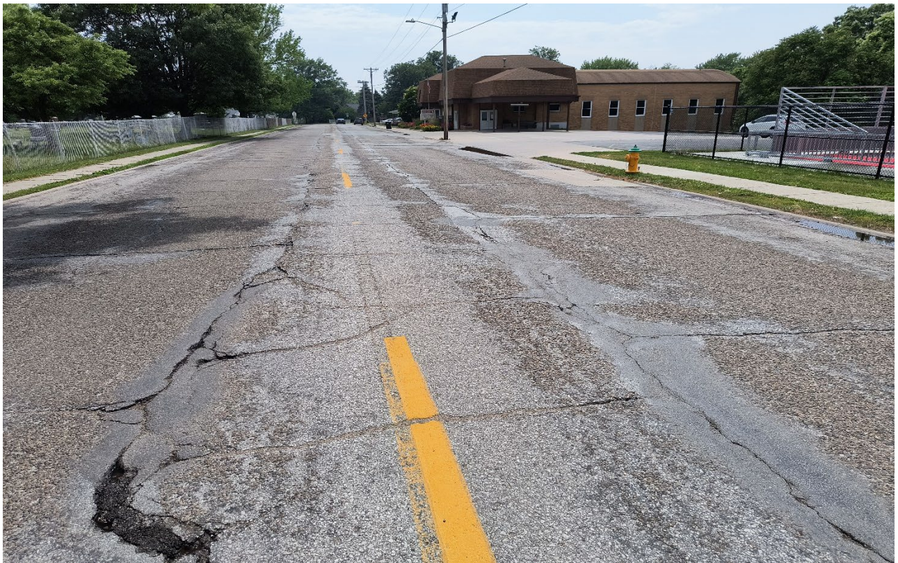
Existing pavement condition. Chip seal was added in the late 90's as an attempt to preserve the asphalt.
