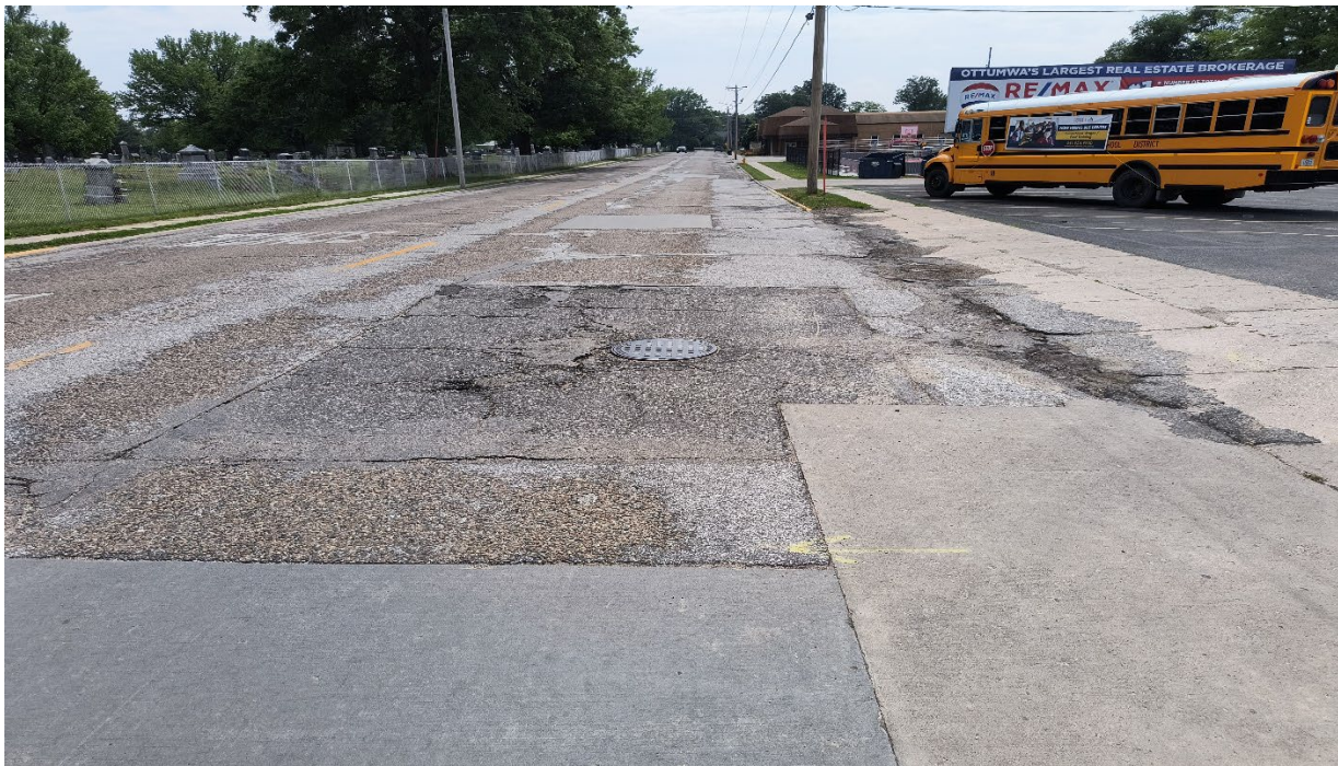
Multiple patching attempts including HMA, and PCC. Failing Gutterline.
